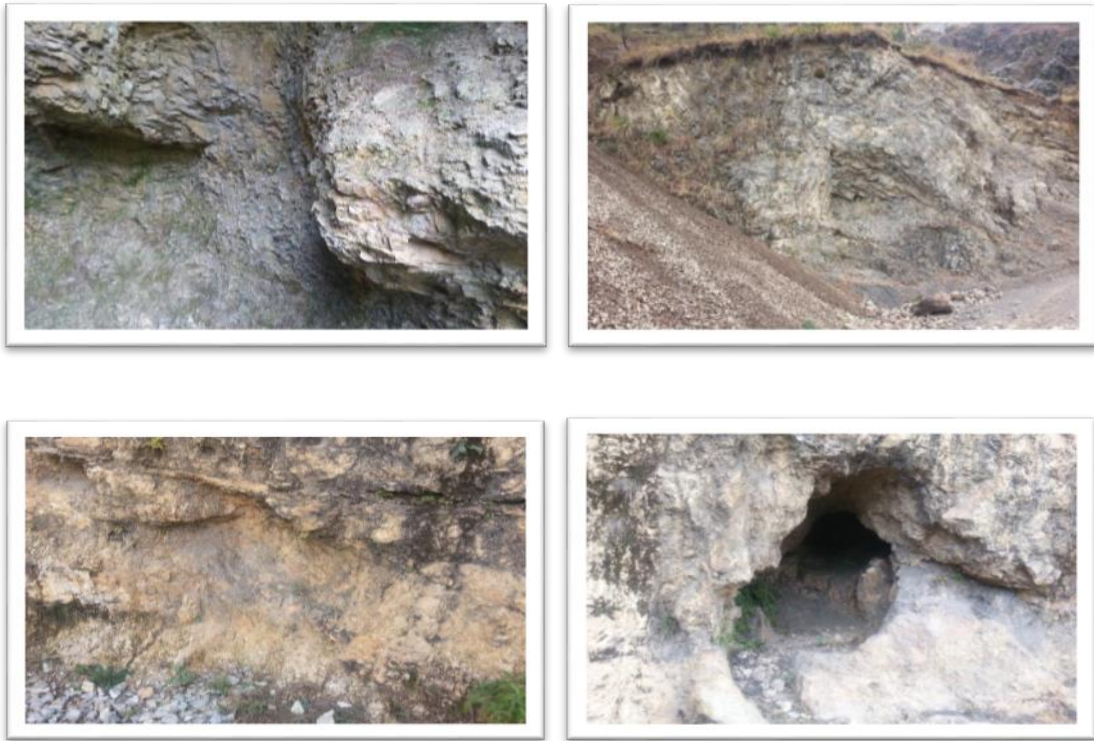
Examples of Trenching in Already Road Cut Section where it was not needed.
